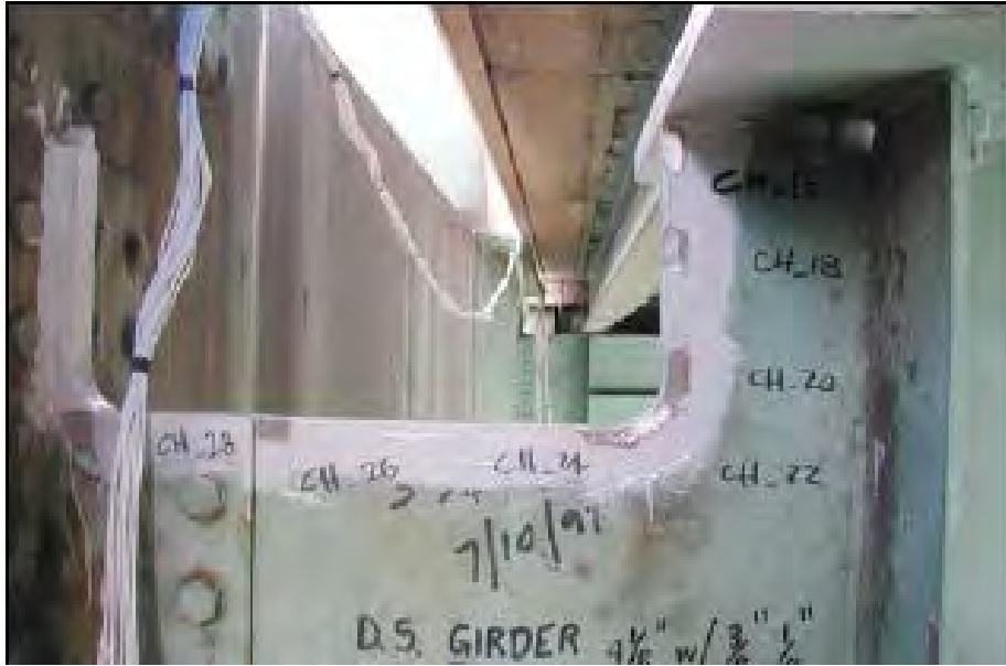
Figure 52. Photo. Tie girder/floor beam connection retrofit on Birmingham Bridge, Pittsburgh, Pennsylvania. Taken from Connor et. al. (87)
