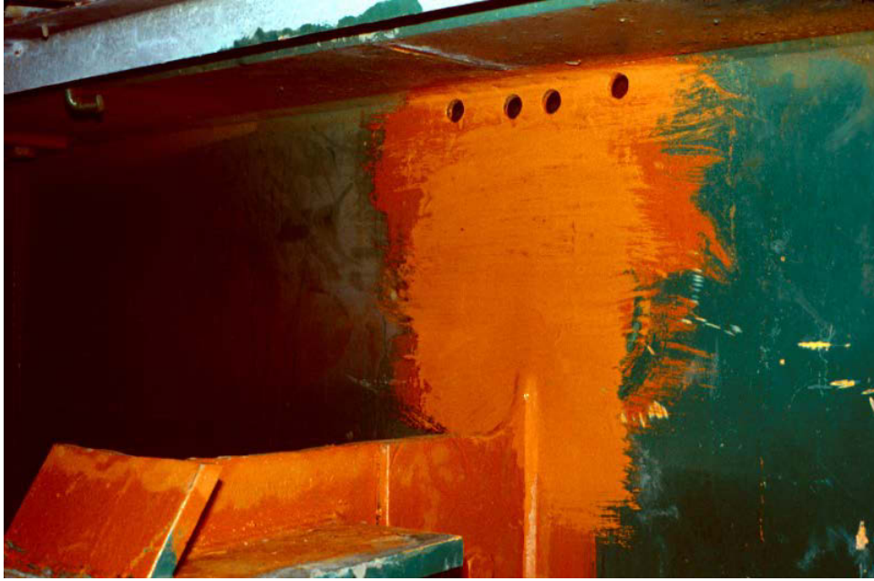
Figure 44. Photo. Completed web gap softening retrofit on Poplar Street Complex. Photo courtesy of Wiss, Janney, Elstner Associates. (82)
