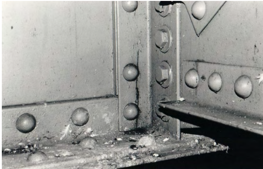
Figure 66. Photo. Cracked connection angle. Photo courtesy of John Fisher.
