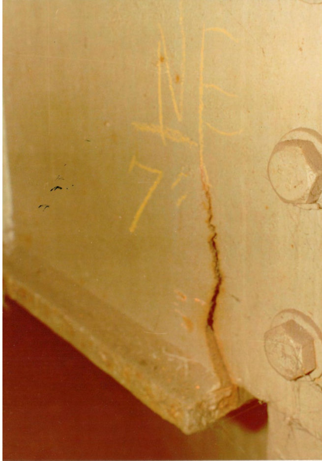
Figure 84. Photo. Close-up view of a crack in a coped beam. Photo courtesy of John Fisher.
