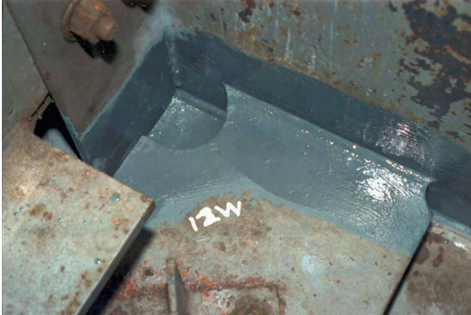
Figure 74. Photo. Completed retrofit of gusset plate weld intersection. Photo courtesy of Wiss, Janney, Elstner Associates.
