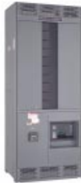
Figure 28: Low voltage switchboard (floor-mounted).
