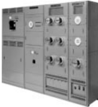
Figure 34: Meter center (floor-mounted).
