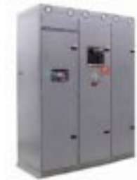
Figure 26: Capacitor bank (floor-mounted).
