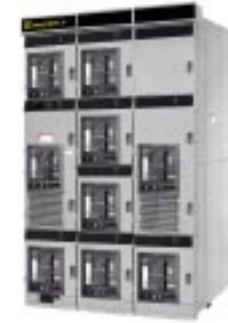
Figure 29: Low voltage switchgear (floor-mounted).
