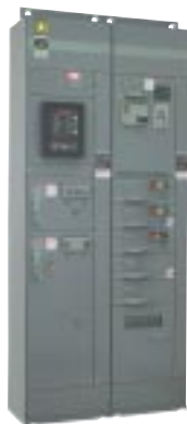
Figure 38: Low voltage motor control center (floor-mounted).
