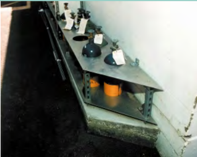
Figure 82: Small gas cylinder storage.
