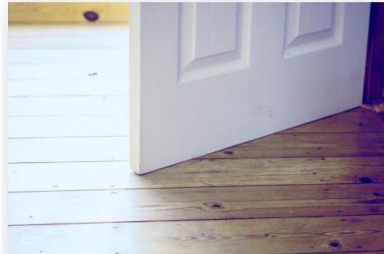
Figure 3. Sticking Windows and Doors
