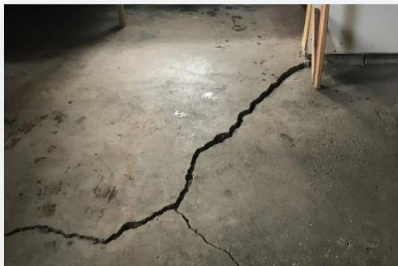
Figure 4. Wall & Floor Damage
