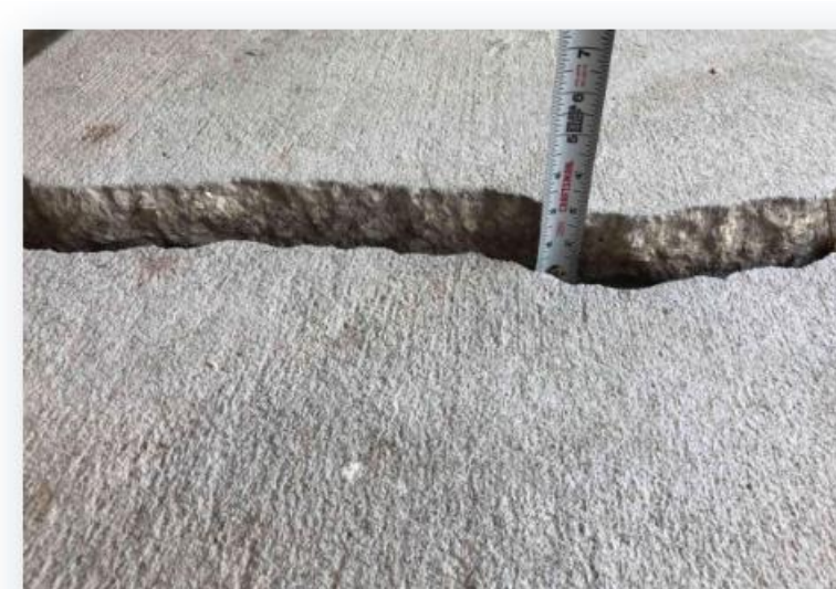
Figure 6. Foundation cracks & deterioration of slabs
