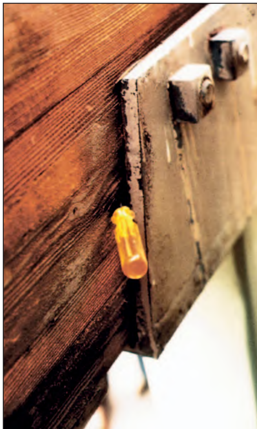
Figure 14-2. Wood decay behind a metal beam connector
