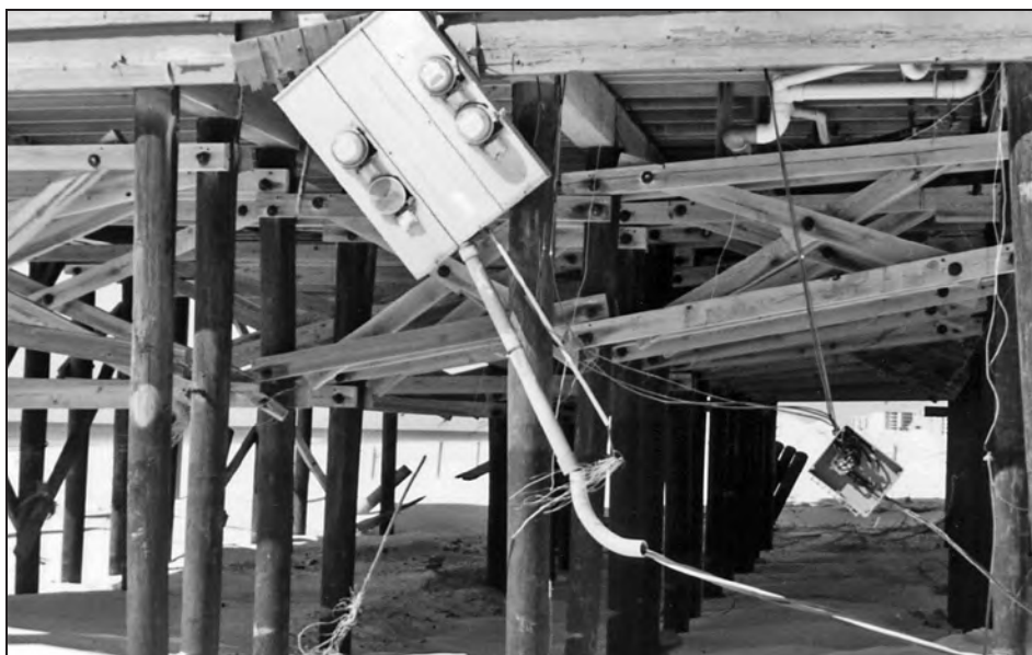
Figure 12-4. Electric service meters and feeders that were destroyed by floodwaters during Hurricane Opal (1995)
