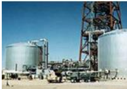
Figure 16: Thermal Storage System
