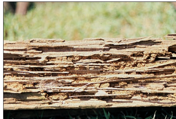
Figure 6. — Wood damaged by subterranean termites.
