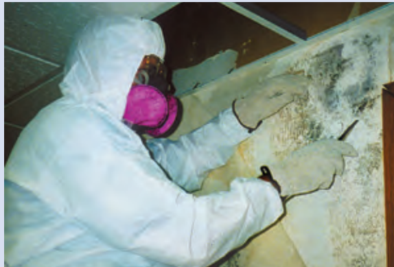
Photo 7: Remediation worker with limited PPE
