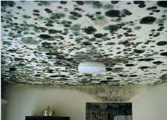
Photo 2: Extensive mold contamination of ceiling and walls
