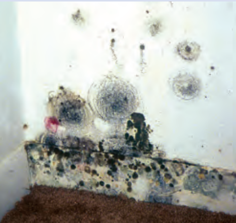
Photo 3A: Mold growing in closet as a result of condensation from room air
