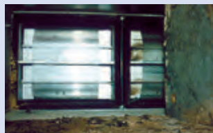
Photo 4C: Moldy air duct
