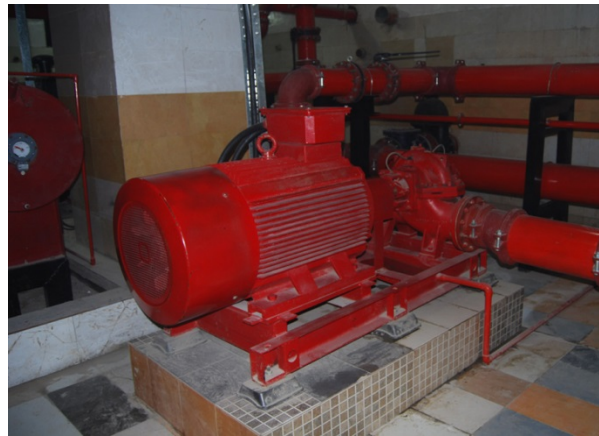
An electric fire pump located in a fire-fighting pump room
