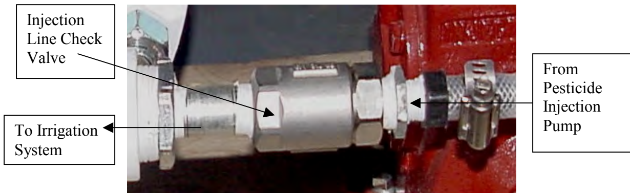
Figure 2: Quick-closing check valve on pesticide injection line
