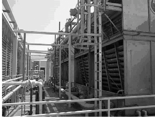
FIGURE 1 COOLING TOWERS FROM A CHILLED WATER COOLING PLANT
