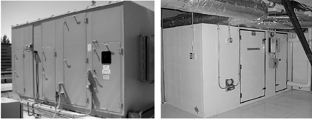
FIGURE 1 INTERIOR AND EXTERIOR AIR HANDLING UNITS
