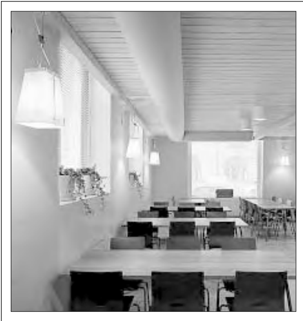
Half-round textile ducts in the Carlsson company's dining room (in Sweden) retain their shape even when not inflated with supply air.
