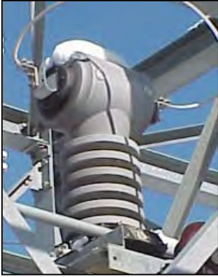
Current Transformer in Switchyard.
