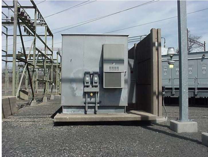
Fig. 13. 138 kV Cable Oil Pump House with a Fire Wall
