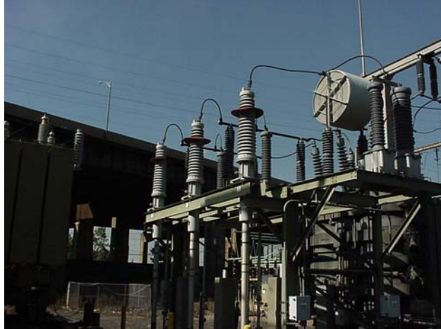
Fig. 16. 138 kV Post Insulators with Creepage Extenders
