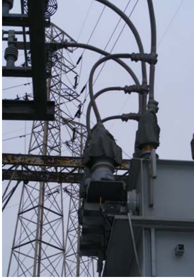
Fig. 17. 13/4 kV Transformer 13 kV Bushings and surge arresters with rubber boots
