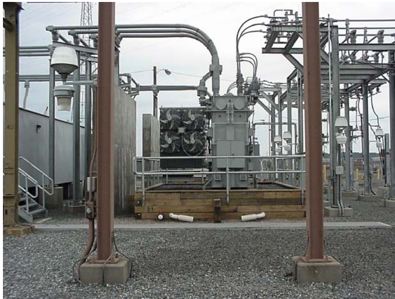
Fig. 3. 13/4 kV 6.0/9.0 MVA OA/FA Transformer
