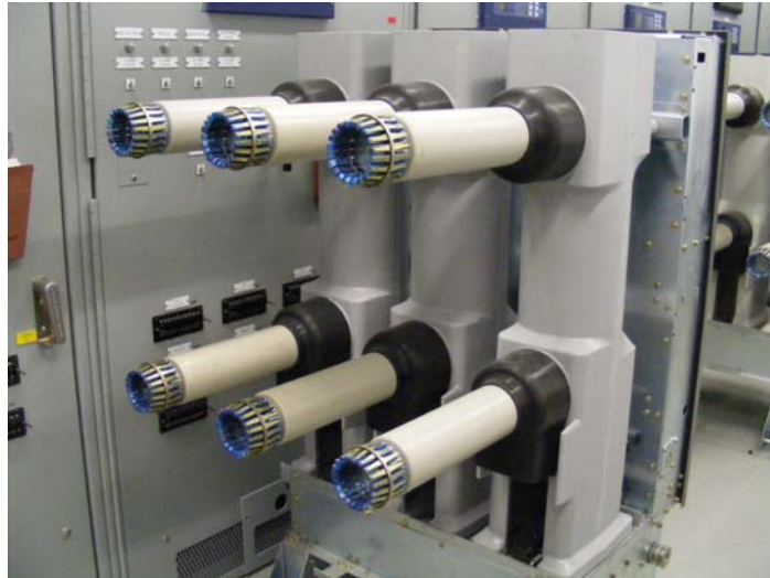
Fig. 7. 26 kV Indoor Switchgear Draw-out Type 2000A Circuit Breaker
