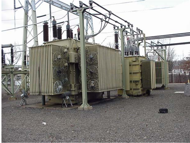
Fig. 4. 138/13 kV 27/36/45 MVA OA/FA/FA Transformer
