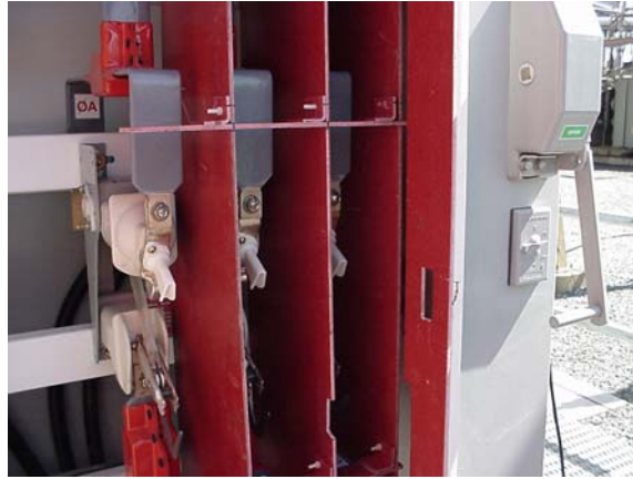
Fig. 10. 4 kV Disconnecting Switch with Insulating Barriers between Phases
