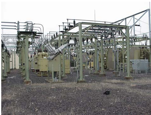
Fig. 6. 26 kV Outdoor 2000 A Circuit Breaker
