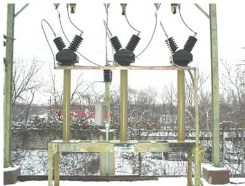
Fig. 21. 26 kV Potential Transformers
