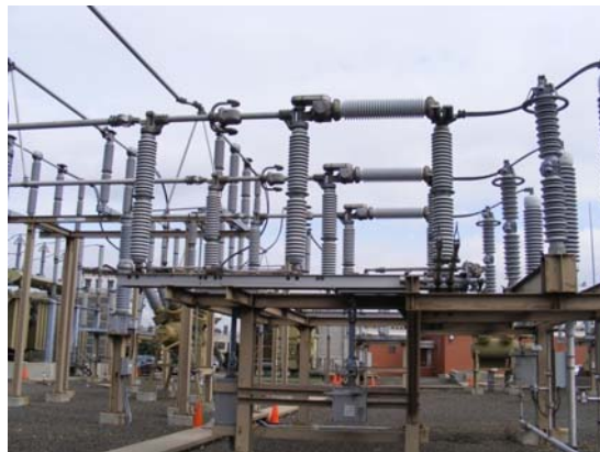
Fig.11. 230 kV 1200 A Circuit Switcher Substation Bus Systems
