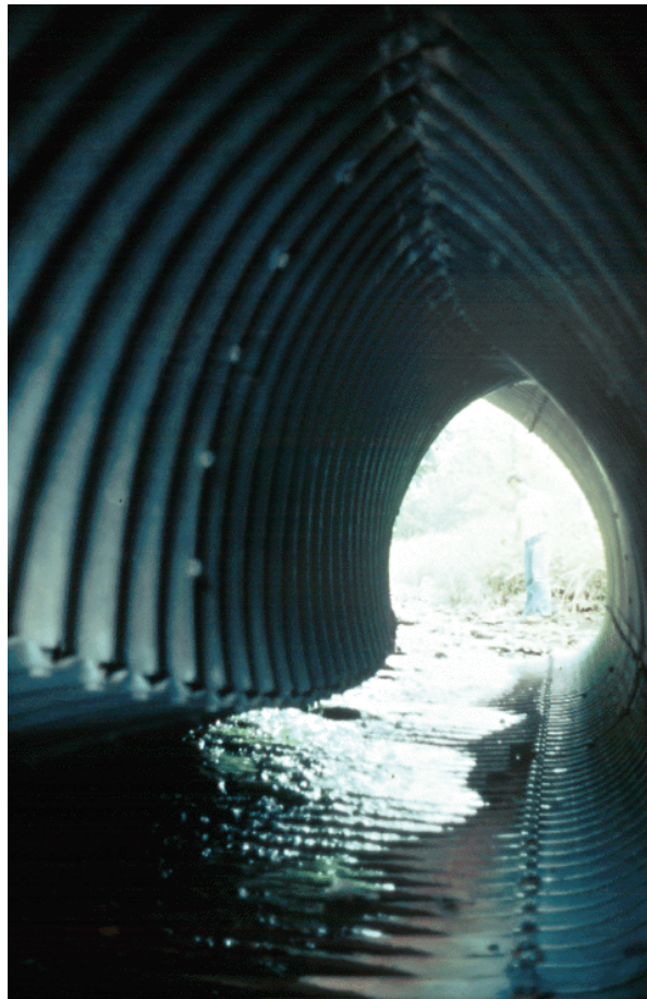
Figure P.3.22 Bending or Shear Failure
