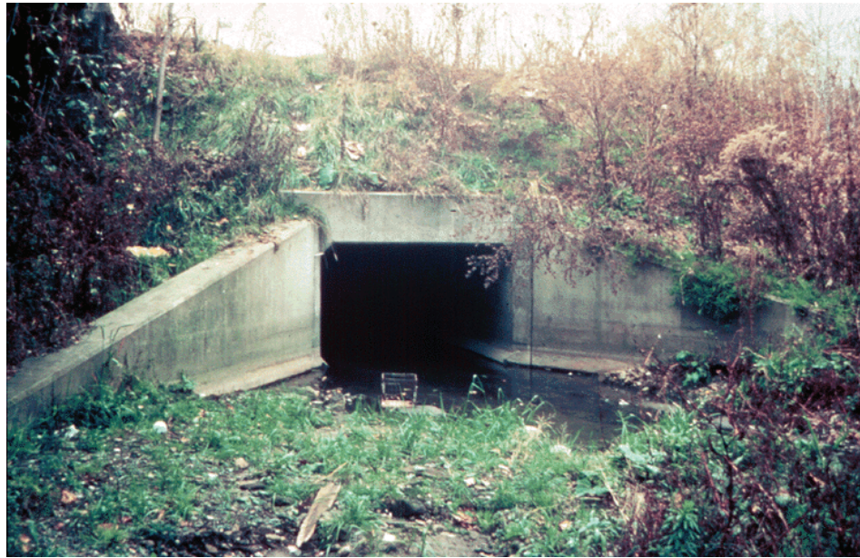
Figure P.3.30 Potential for Tilted Wingwalls
