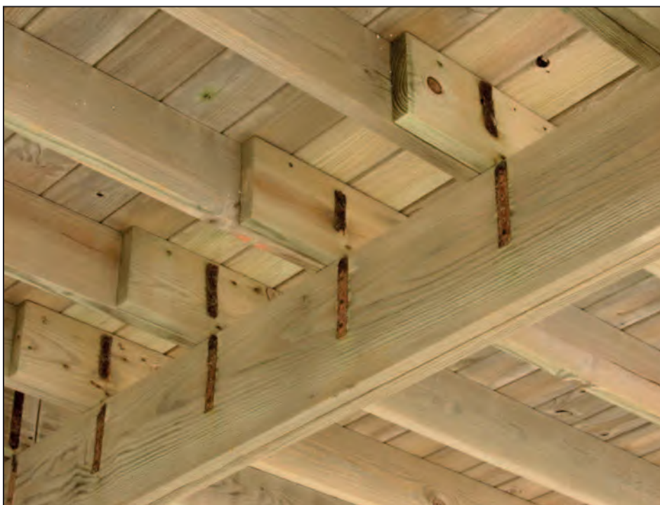
Figure 14-3. Severely corroded deck connectors
