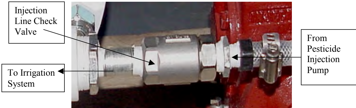
Figure 2: Quick-closing check valve on pesticide injection line
