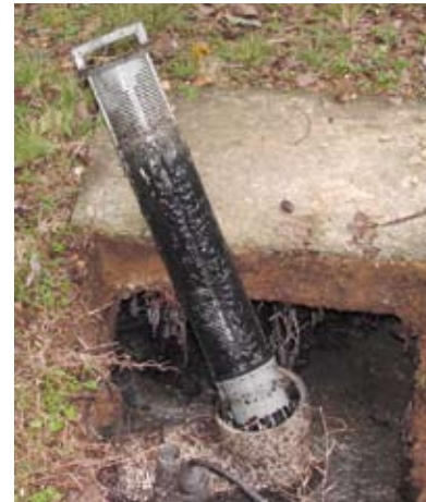
System inspections are a key component of management programs. Clogged septic tank effluent filters (above) can trigger calls for needed service, but regular inspections tailored to system type, setting, and use profile provide a better approach for ensuring long-term system performance.
