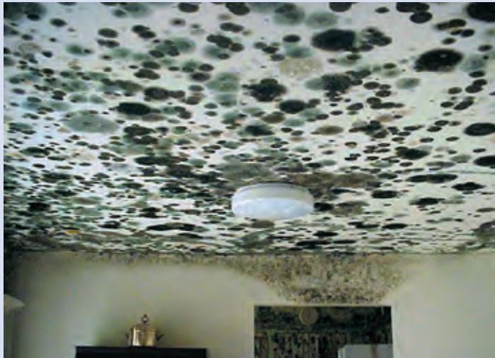
Photo 2: Extensive mold contamination of ceiling and walls
