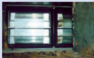
Photo 4C: Moldy air duct
