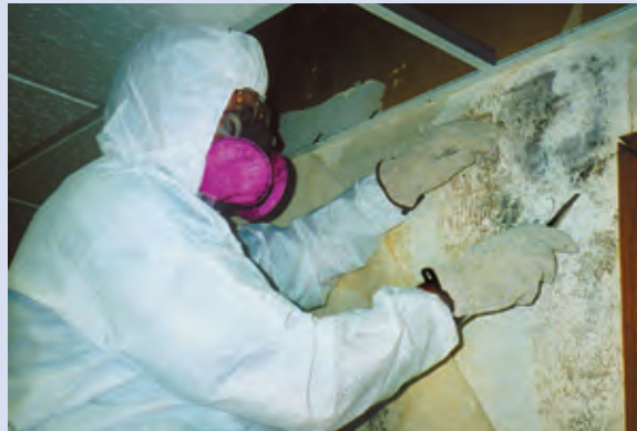
Photo 7: Remediation worker with limited PPE
