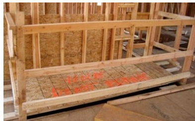
Covered floor hole marked, and with a guardrail surrounding it.
