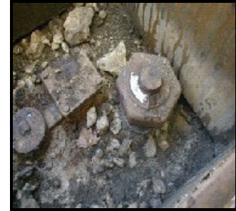
Equipment and metal piping covered with dirt in uncontained sump
