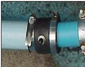
Test boot located in a sump
