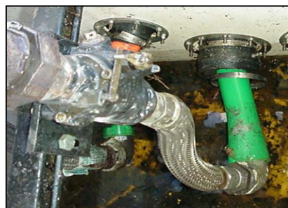
Metal flexible connector is twisted due to growth of flexible plastic piping
