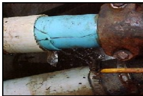
Flexible piping is cracked
