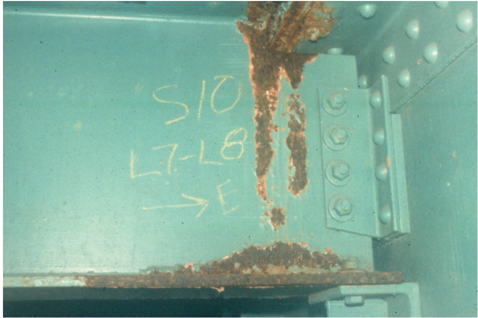
Figure 8.6.55 Corroded Stringer Connection
