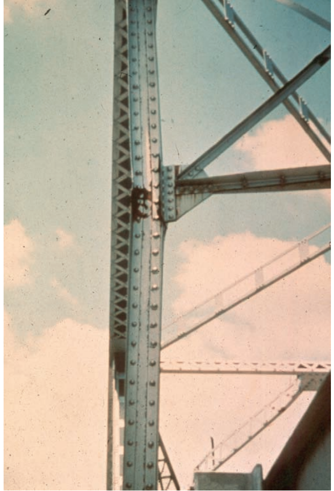
Figure 8.6.51 Collision Damage to Vertical Member
