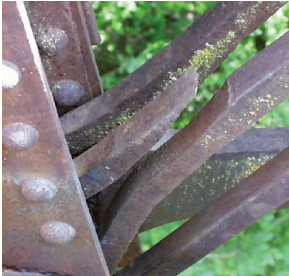
Figure 8.6.46 Cracked Forge Zone on a Loop Rod
