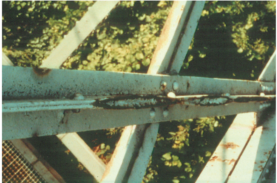
Figure 8.6.66 Sway Bracing with Rust Packing
