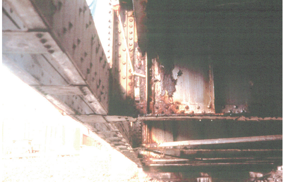
Figure 8.6.53 Corroded Floorbeam End and Connection
