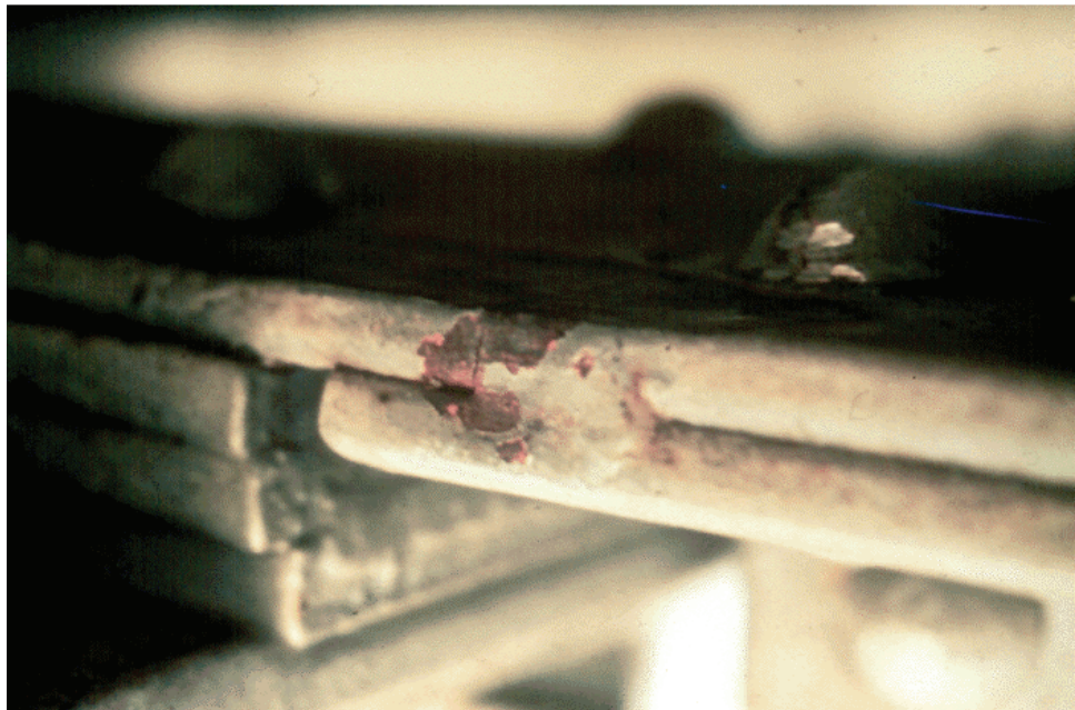
Figure P.1.21 Close-up of Tack Weld on a Riveted Built-up Truss Member
