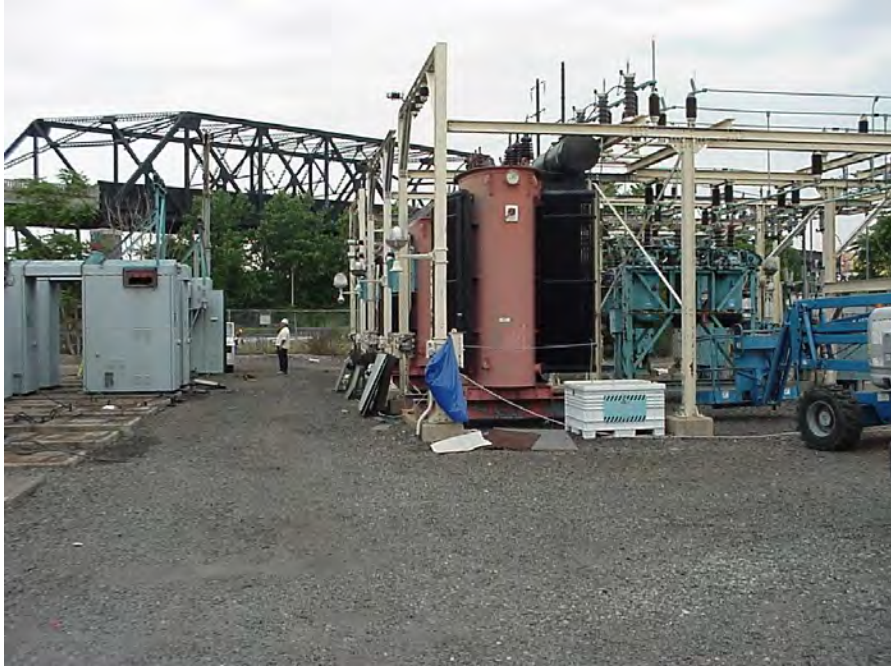
Figure 4 - Main Street Substation before Renovation
