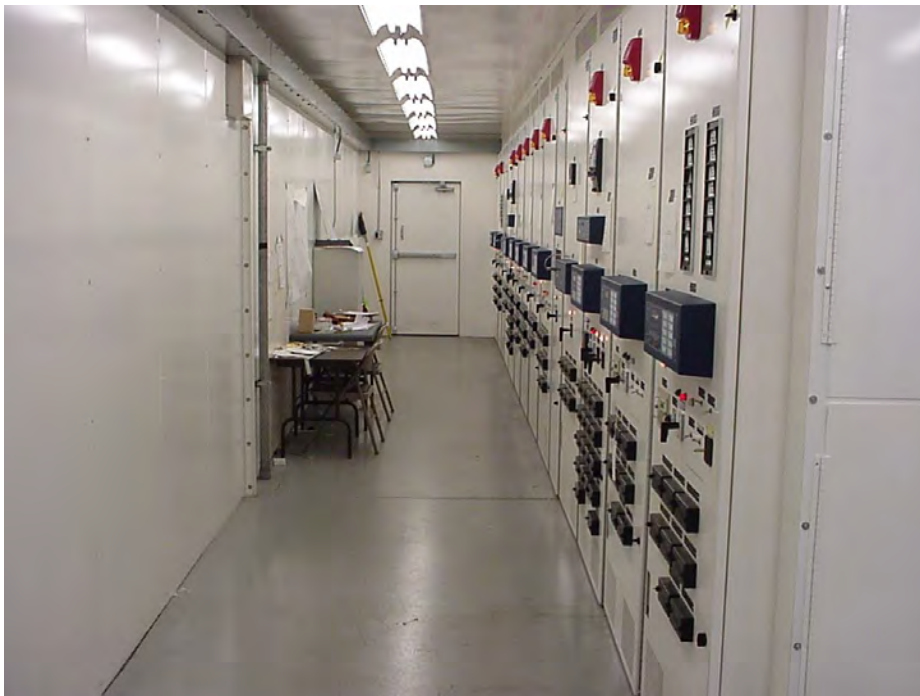
Figure 7 - Metal Enclosed 4 kV Switchgear [Inside View]
