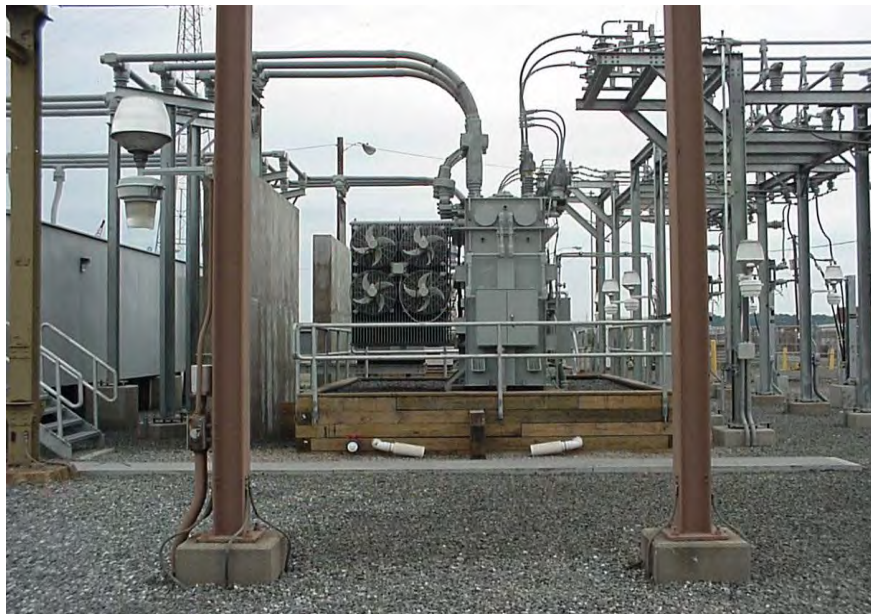
Figure 5 - New 13/4 kV Transformers and 13 kV Switchyard
