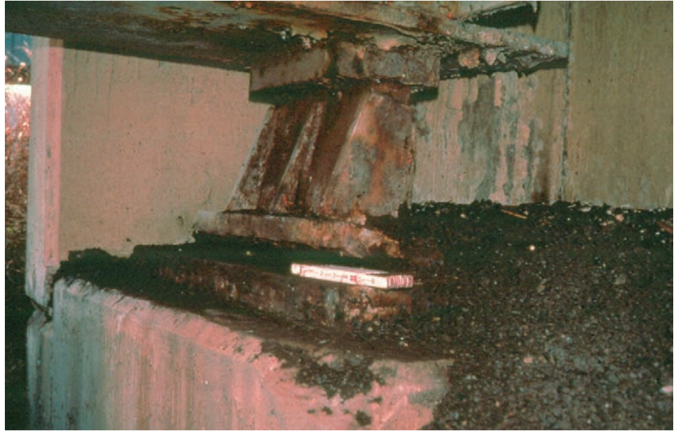
Figure 9.1.22 Heavy Corrosion and Excessive Movement on Steel Rocker Bearing
