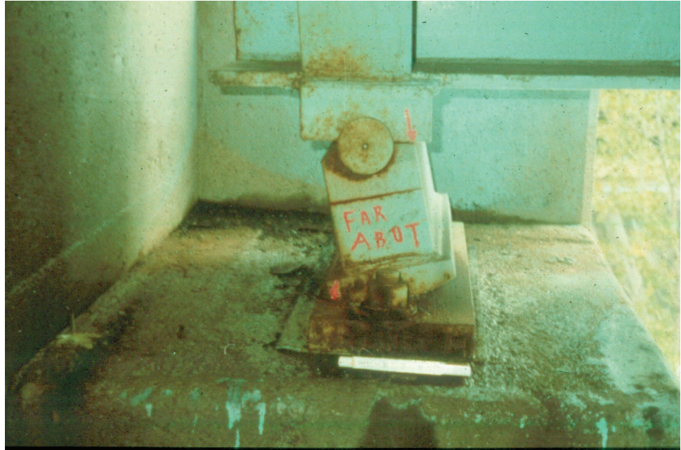
Figure 9.1.38 Broken Pintle on a Bearing
