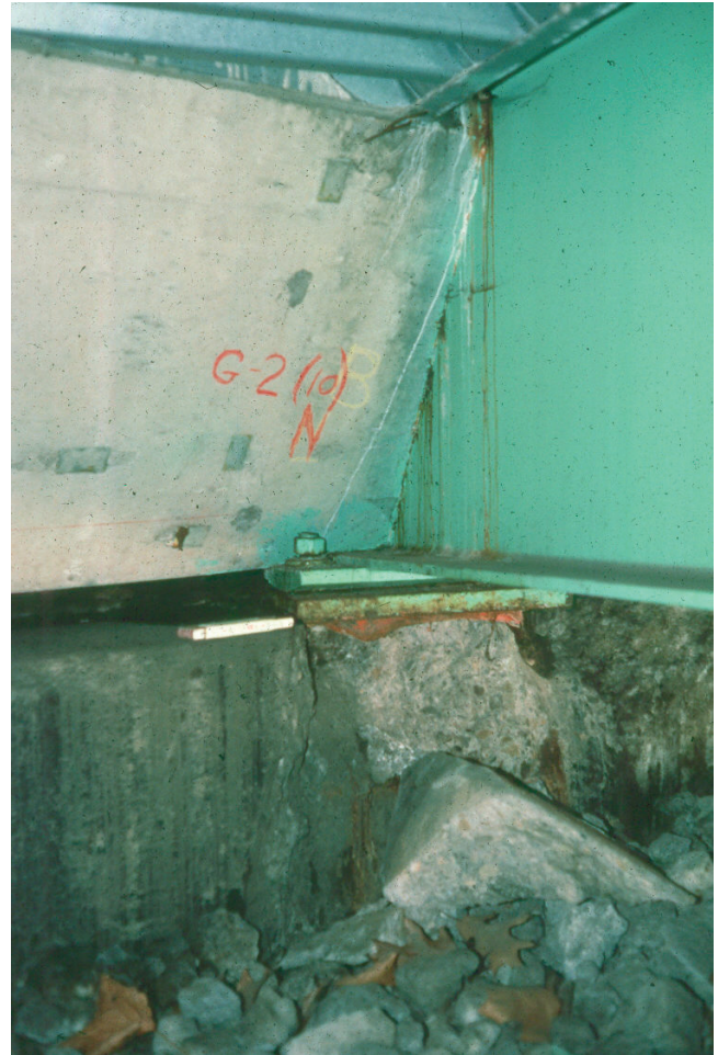
Figure 9.1.24 Spalling of Concrete Bridge Seat Due to High Edge Stress
