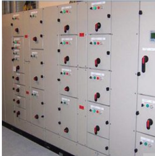
A Typical Motor Control Center
